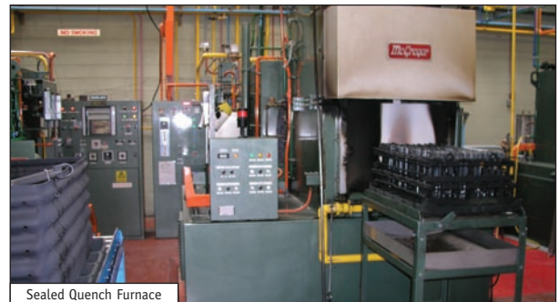
Sealed Quench Furnace
